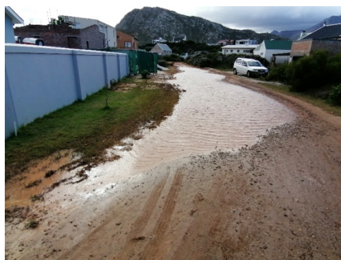
Much of the unsurfaced road network within Pringle Bay is unsurfaced and poorly drained. There is frequent flooding of low-lying areas of the village
